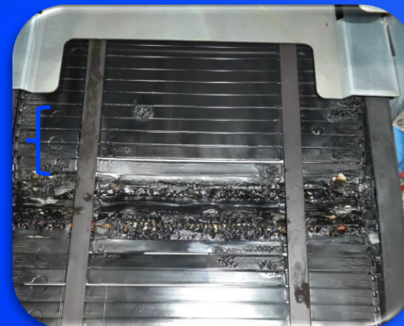
Thermal runaway limited to 4 cells
