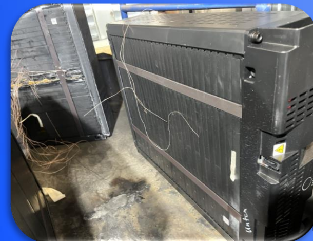
Adjacent battery modules not damaged
